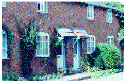
Lean-to canopies on brackets, Welford-on-Avon, Avon Valley area. The roof material in this case is inappropriate
