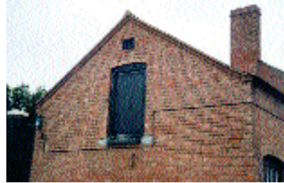
A trim verge of brick with slate undercloak, a projecting stretcher course and a simple angled ridge tile in Lower Quinton, Avon Valley area
