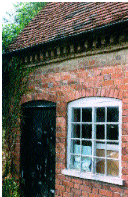
Variation of dentilated brick eaves with alternating projecting headers on edge, also showing a rise-and-fall gutter fixing, Great Alne, Arden area
