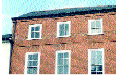
Gauged brick flat arches on a house in Henley-in-Arden, Arden area. The openings are vertically aligned and the second floor windows are smaller than the first floor windows.
