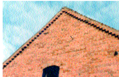
A trim verge of brick with stepped projecting header corbelling and a half-round ridge tile in Alcester, Arden area
