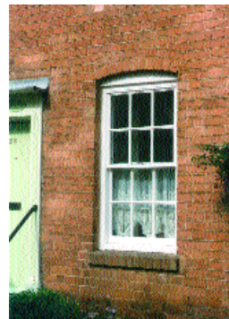
A window with a segmental arch head in Alcester, Arden area. Note that the arch is made up of one course of headers on edge and one course of headers laid flat, a detail very characteristic of brick areas within the District.
