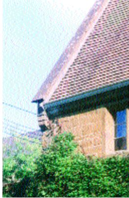
A stone-coped gable parapet of Hornton stone with a corbelled verge/eaves junction known as a kneeler. Avon Dassett, Cotswold Fringe area
